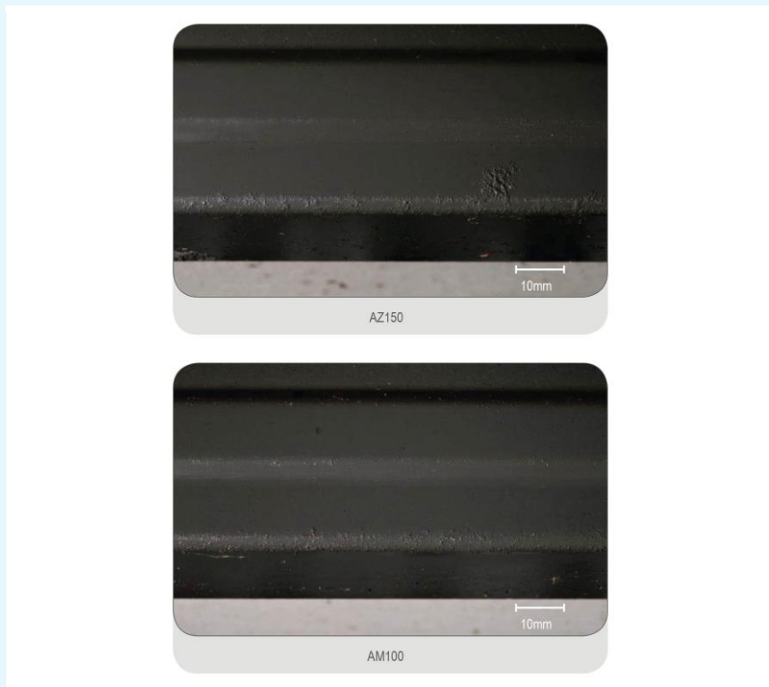
Figure 7: Prepainted, sheltered fascia bends (i.e. unwashed) after 57 months exposure within 100m from breaking surf on an outdoor test facility.
