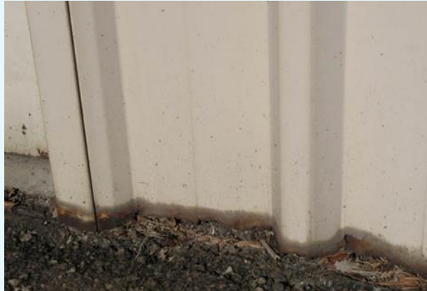
Figure 2: Corrosion due to inappropriate wall design
