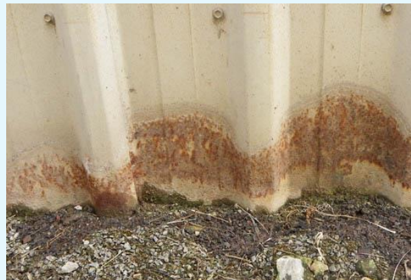
Figure 3: Corrosion due to immersion in soil
