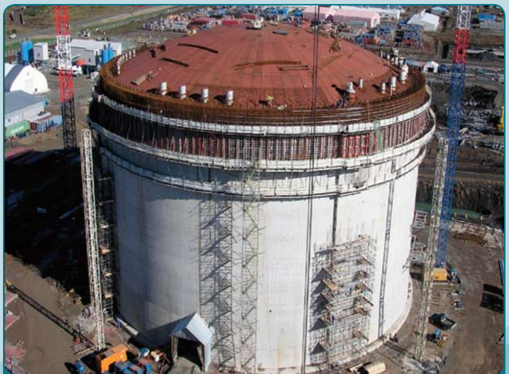
Huge LNG tanks like this will hold gas from the Pluto field.
