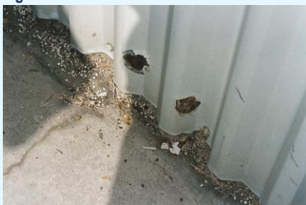
Figure 1: Corrosion due to fertiliser contact
