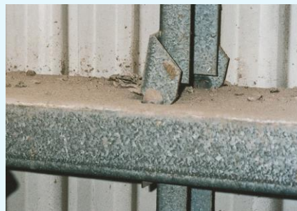
Figure 2: Build-up on purlin
