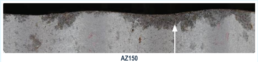
Figure 2: Unpainted sheltered walling (i.e. unwashed) in a severe marine environment after 50 months.
